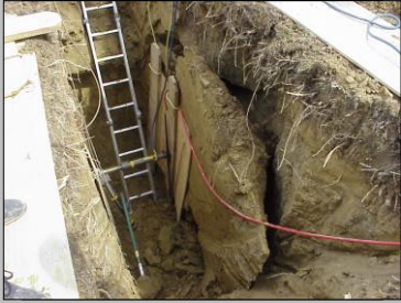
Slough or Belly Failure
